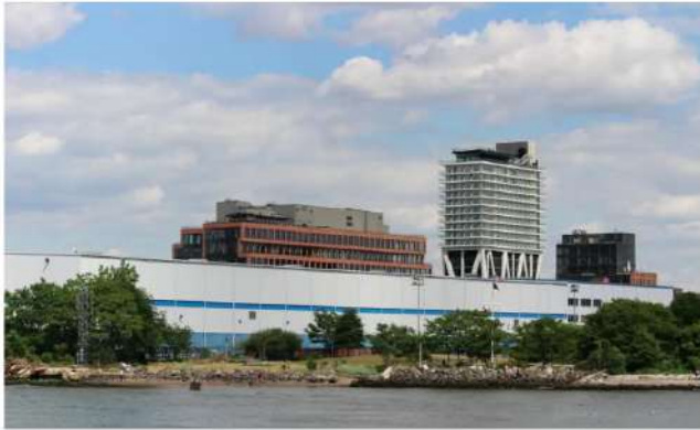
The CitiStorage building at Bushwick Inlet Park, shown in June of this year, is set to be totally demolished by the end of the year. Photo by Susan De Vries
